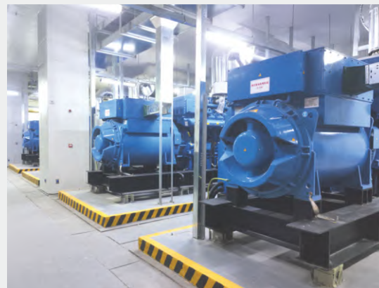
■ China Telecom (Beijing-Tianjin-Hebei) Big Data Industrial Park
