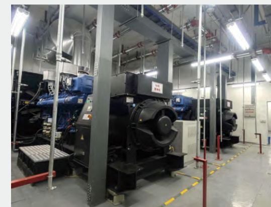
■ China Telecom Lanzhou New Area Big Data Industrial Park
