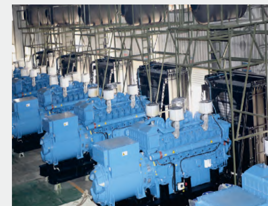
■ China Telecom Smart Cloud Base Huailai Park
