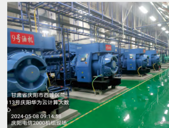
■ China Telecom Qingyang Computing Power Center (National Hub of "East Data, West Computing")
